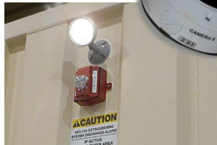
Security system installed & tested
