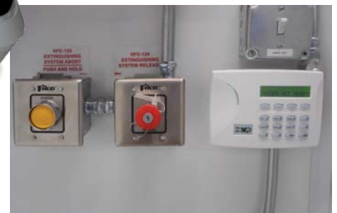
Clean agent system installed & tested
